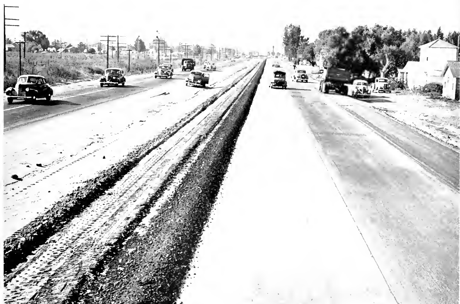
Divided highway unit of U. S. 99 nearing completion south of Modesto with traffic using outside lanes
